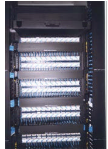
Rack Rear Detail
